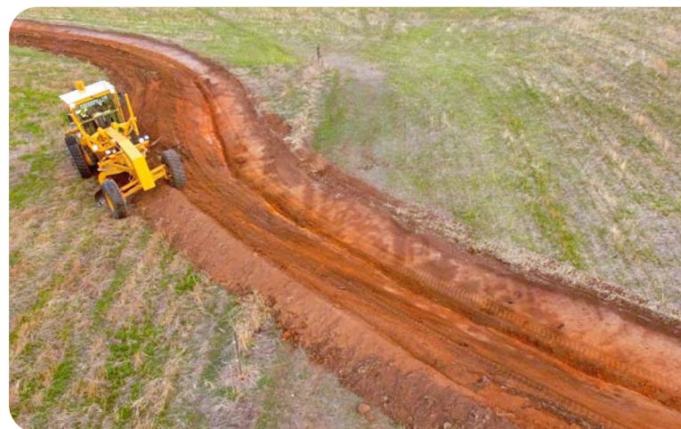
Contour being installed in Boyup Brook, WA.
