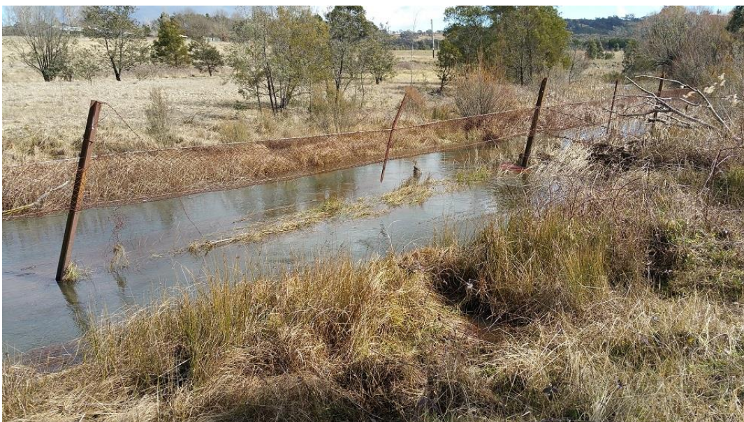
Figure 9 – In all cases, willow revetments constructed during the 1970s are now undermined.
